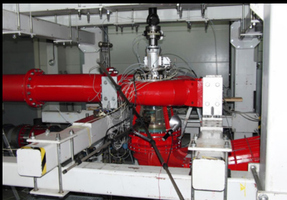
HPP Lower Baker / USA
